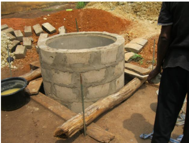
Prototype of water well under construction Cement blocs are made on site
