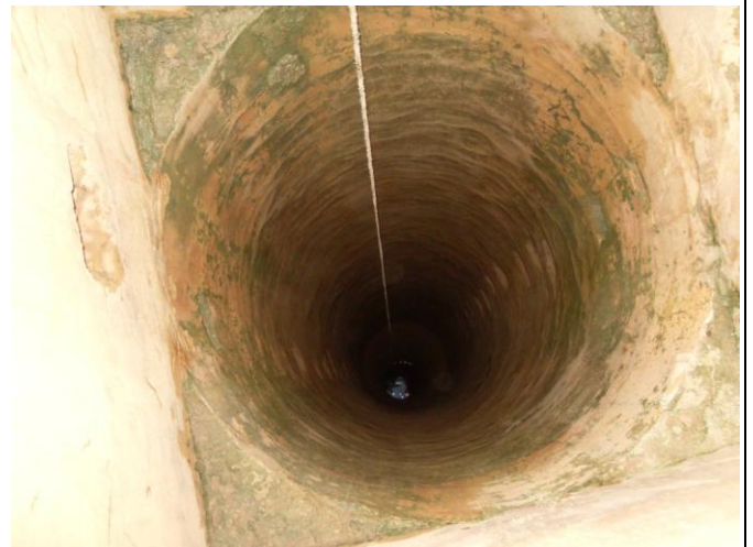
An operational well in Lomé
